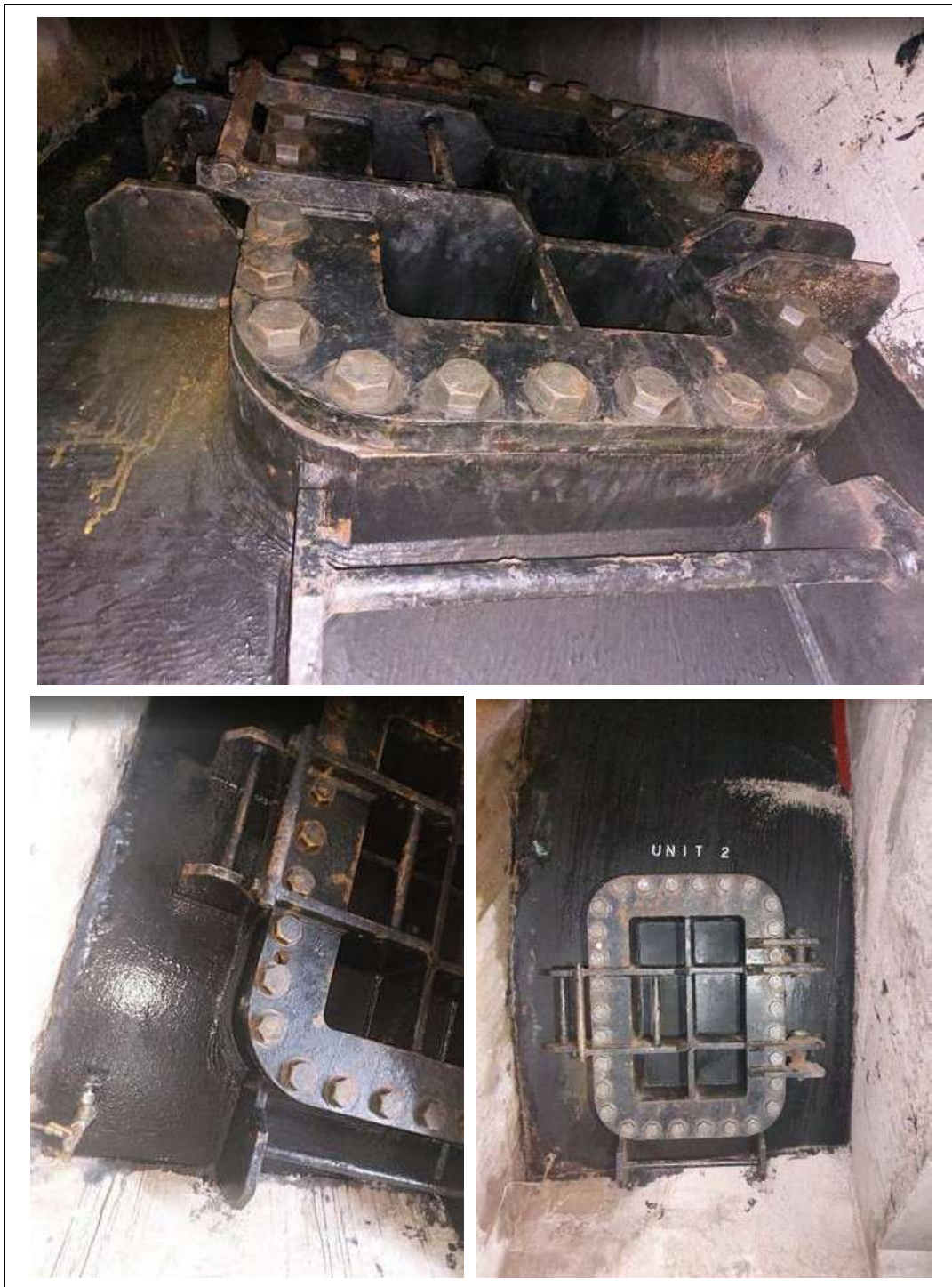
Figure 11: Spiral casing access mandoor in closed/sealed condition with spiral casing filled
