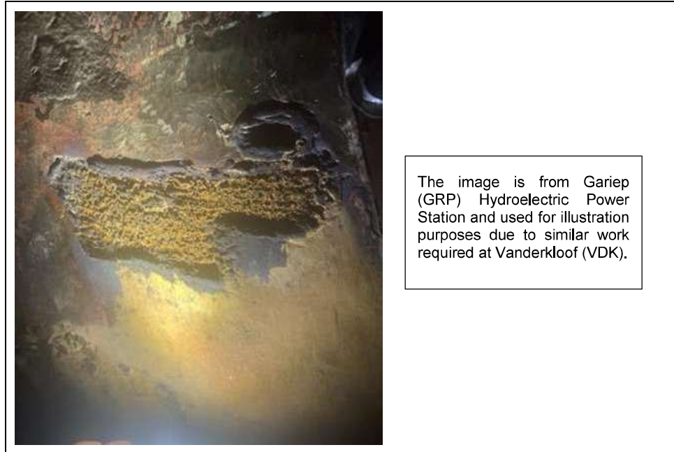
Figure 12: Draft tube liner damage
